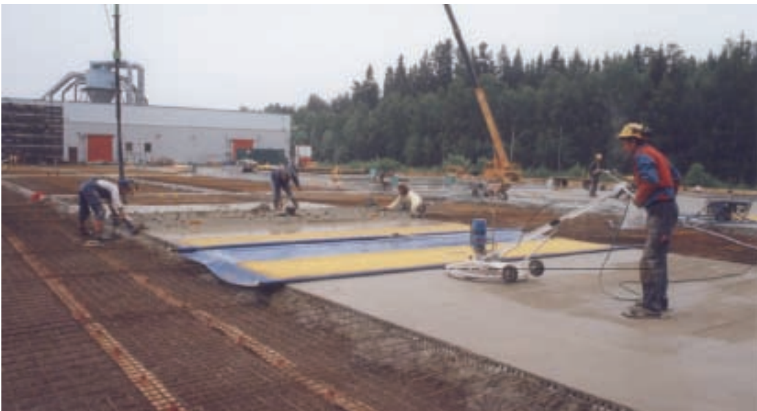
Fig. 4 While vacuum is on, the surface that has already been vacuum dewatered is floated with a power trowel fitted with a disc.
