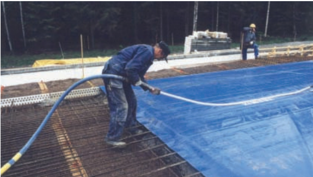
Fig. 3 The top cover is connected to the suction hose of the vacuum pump. Thereafter it is important to check that the top cover seals against the fresh concrete outside the filter pads.
