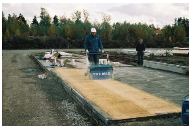
The Tremix Hardtopping material is spread on the still humid concrete surface.
